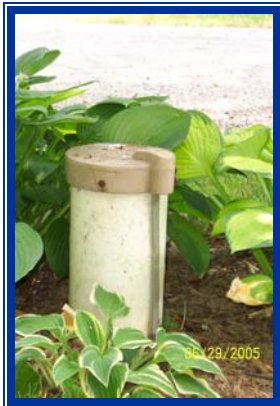
Well cap installed without conduit.
