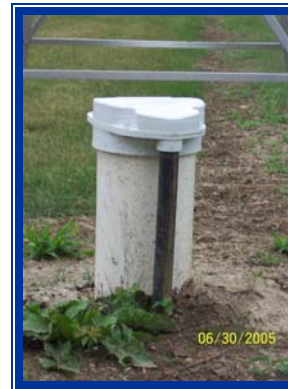
Well cap installed with incorrect conduit material
