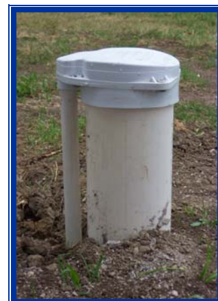
Correct cap and conduit installation
